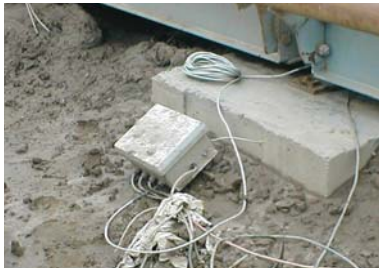
Eliminating junction boxes eliminates a common cause of scale failure.
